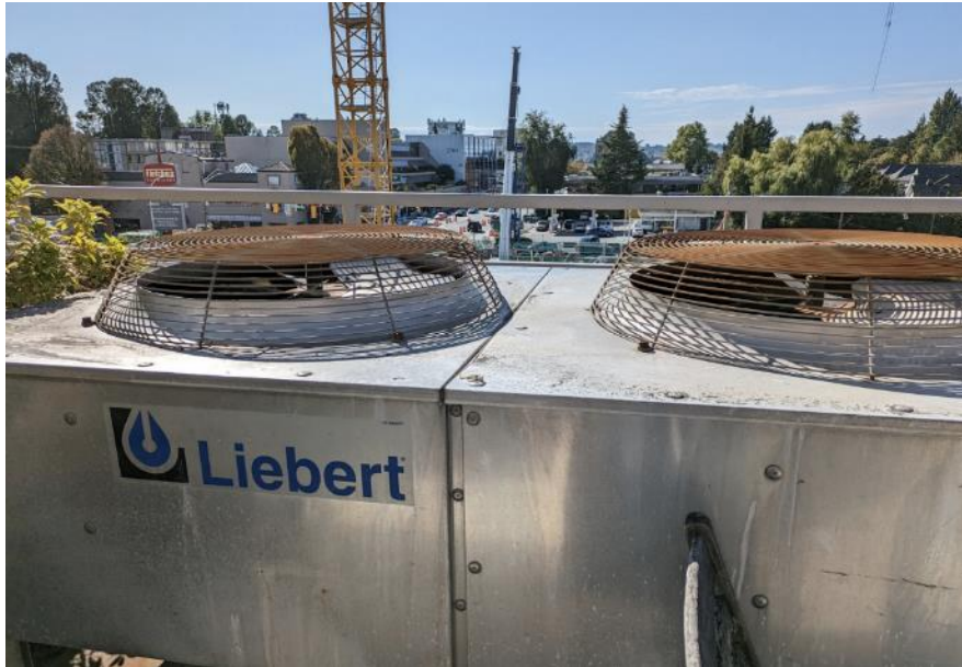
Figure 3.7: External condenser unit
