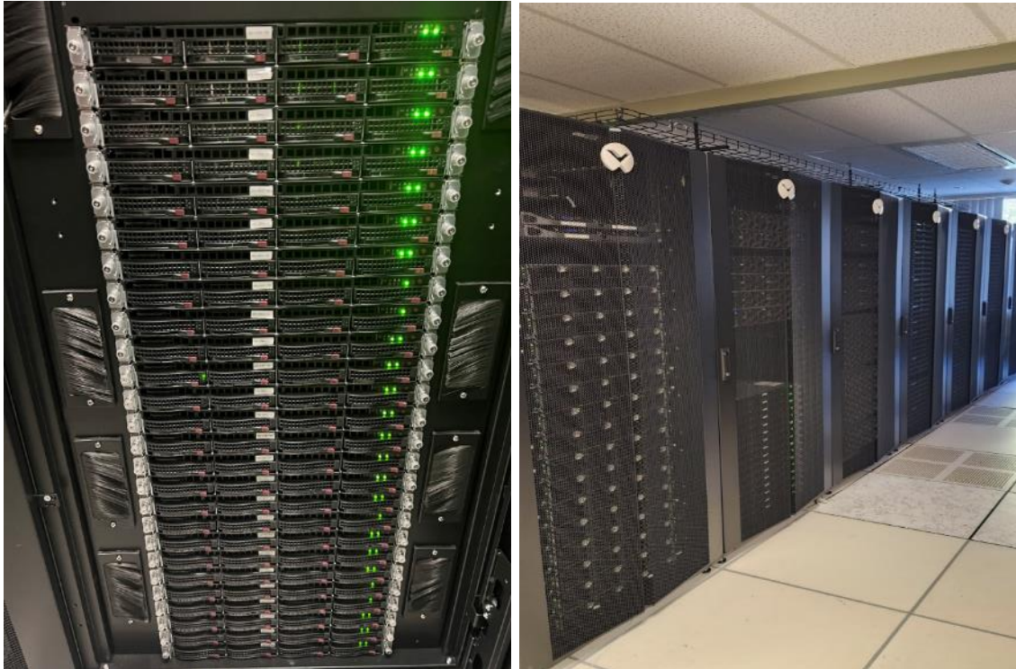
Figure 3.3: Images of sample rack with mounted workstations, and data centre. Each green light is a workstation. There are 27 racks in the data server room. Racks vary in the type and amount of equipment they host.
