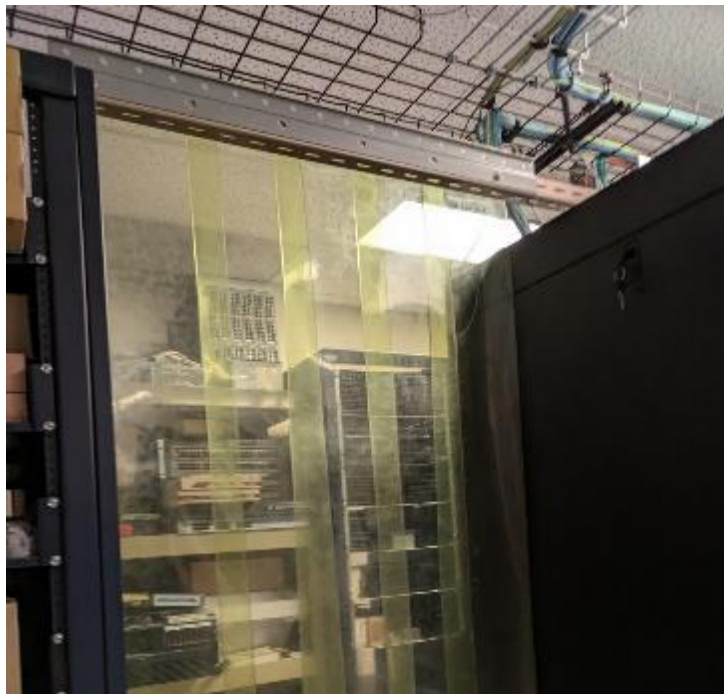
Figure 3.6: Plastic partition between cooling equipment and remainder of data centre.
